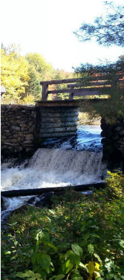
BOTTOM: the Maine Forest and Logging Museum looks forward to having safety railings fully across the Blackman Stream dam.
